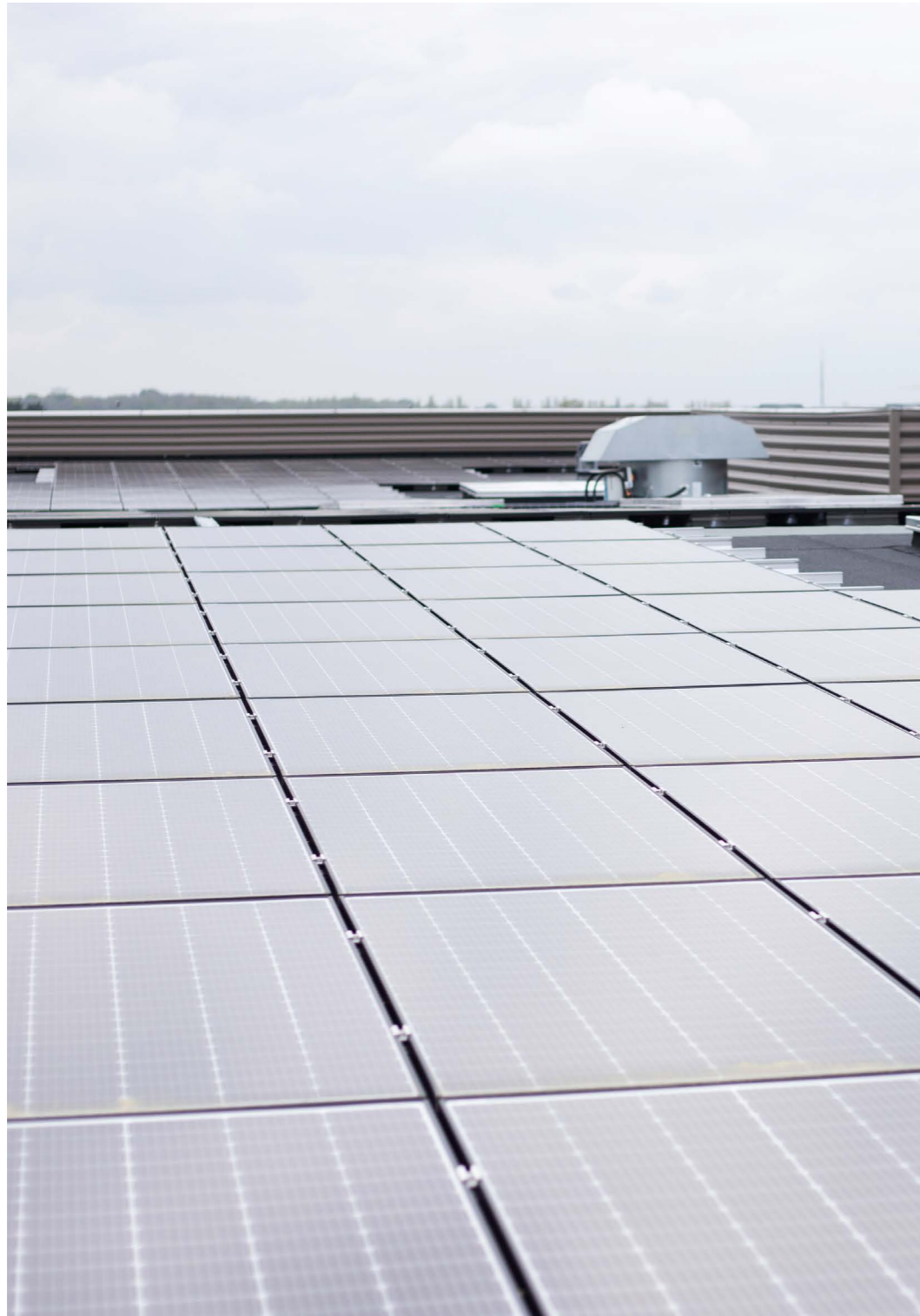
Solar panels at Gainerie 91 France site
